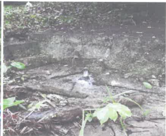
Tubod Spring-Intake Box.
