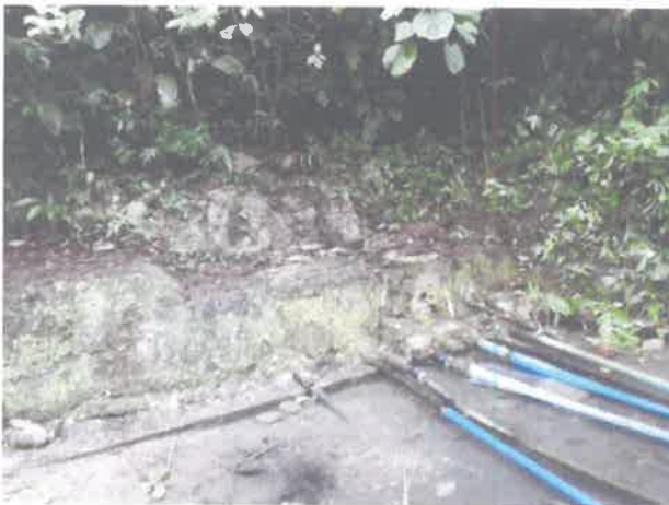
Tubod Spring-Intake Box.
