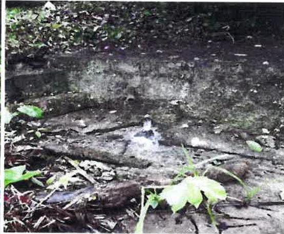
Tubod Spring-Intake Box.
