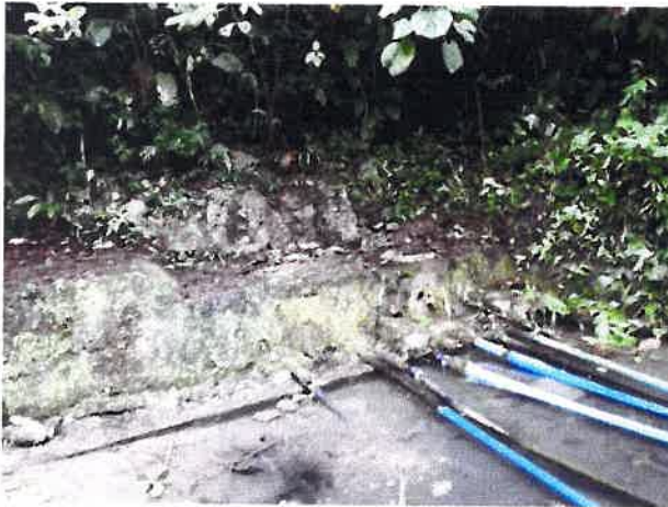
Tubod Spring-Intake Box.
